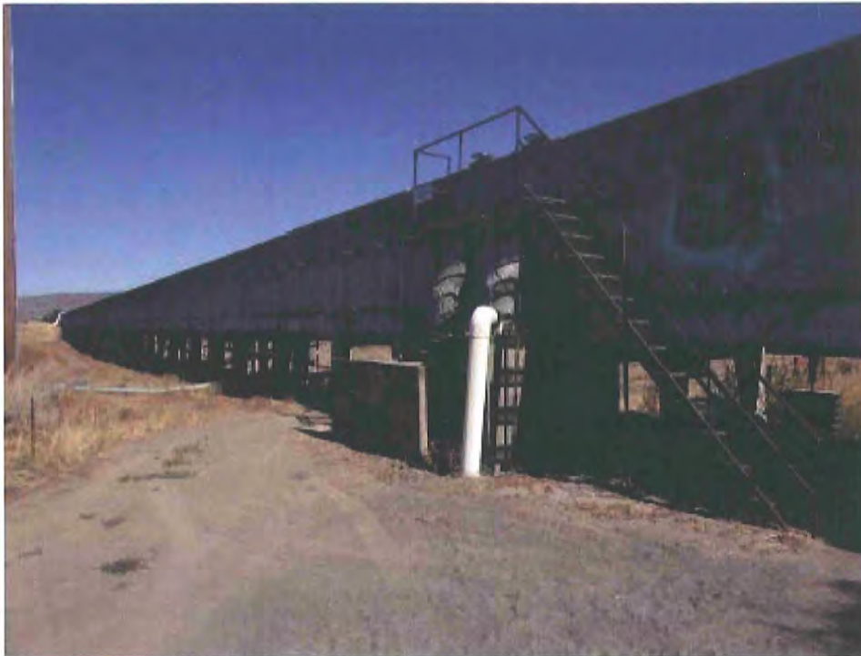
(Photo 7) Termination of the C Flume on the south end of the looking north (LRDC crossing is in the distance)
