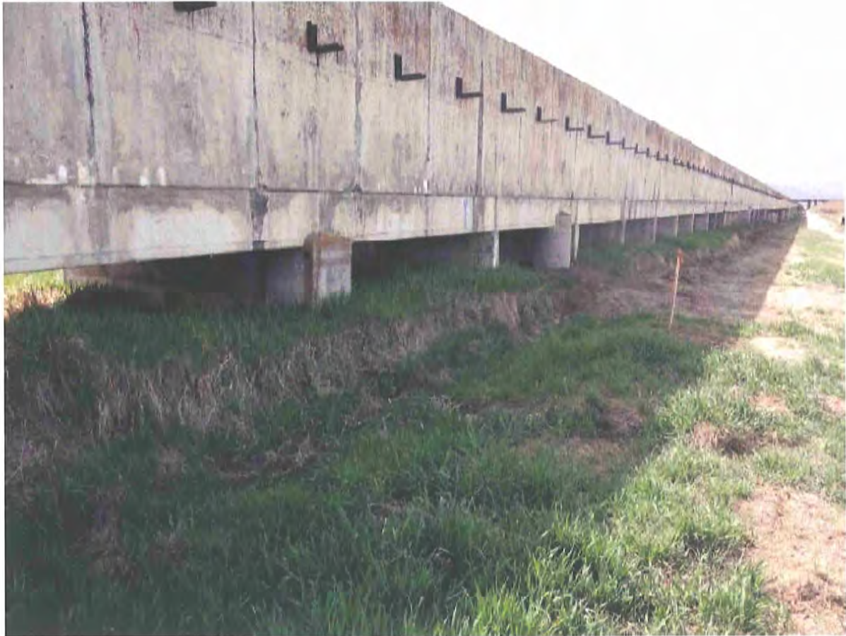
(Photo 1) View southwest of the C Canal Flume (Near the upstream end)
