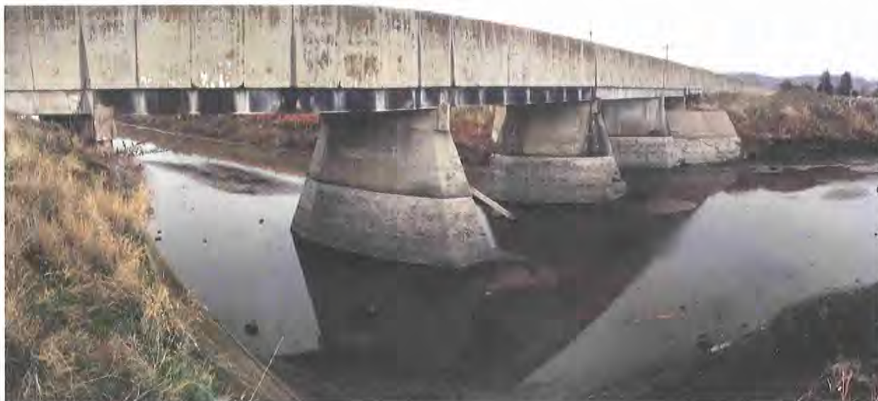
Photograph 1. During drawdown of the Lost River Diversion Channel in November 2014, shallow water remained in the channel near the C Flume Crossing.
